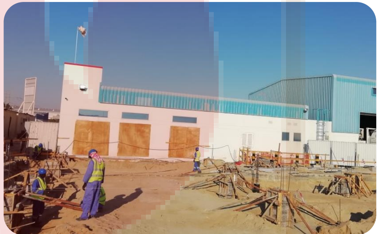
Project: Proposed G+1 Office Building for M/S Air Liquide Global Helium FZE at JAFZA, Dubai.
